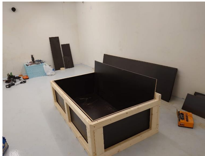
Figure 6 - Sump tank during construction, the inside of the tank was later coated with a rubber sheeting.
