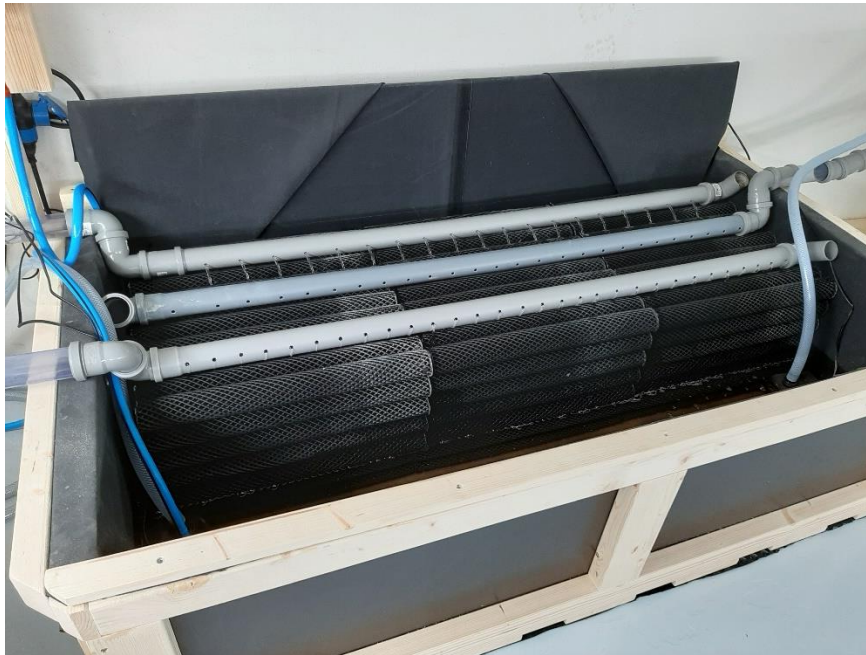
Fig. 10 – Biofilter installed in the sump tank. The biomodules chosen are used for on-site wastewater systems.
