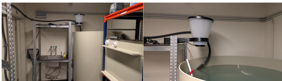
Figure 6. Water supply system and newly built electricity circuit lines and fuse box.
