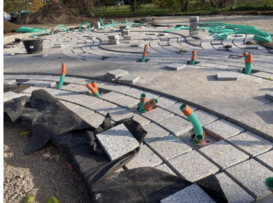
Construction of the above-ground part of the fountain. The green tubes are the nozzle tube ends.
