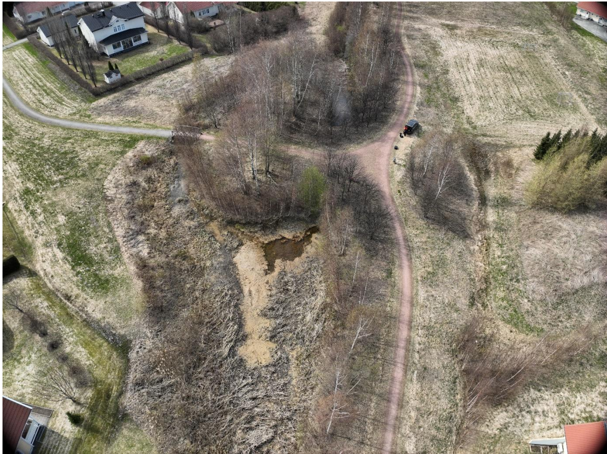
Wetland after the clearing of overgrown vegetation and before construction in May 2024.
