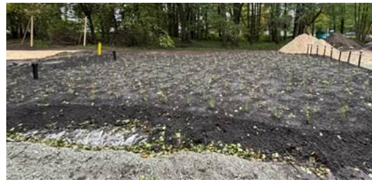
Soil filter after two pond system.
