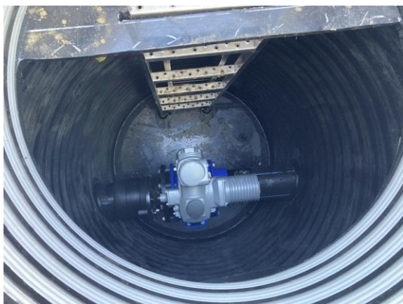
Designed automatic water flow regulation valve on the pond outflow pipe.
