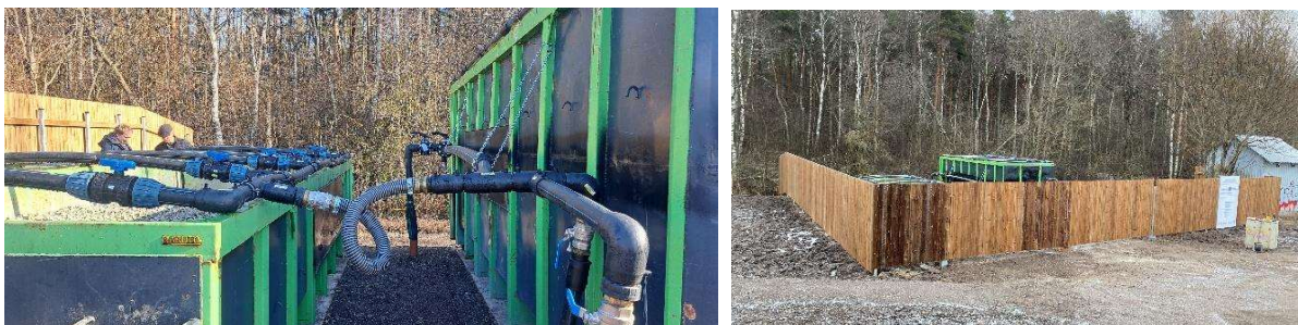
Figure 4.3. Filter system pipe connections and fencing around the site
