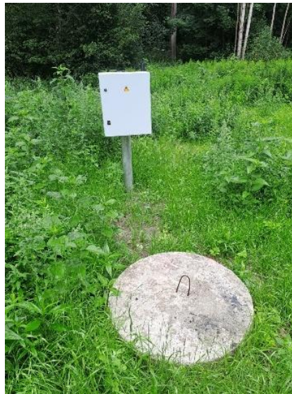
Figure 40. Sensor Power Connection and Monitoring Well
